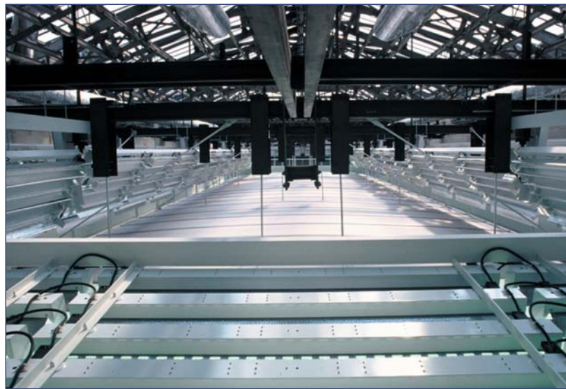
Longitudinal view of the framework: above, the glass roofing is supported by a metal frame. Below the framework, the 16 mm Danpalon filter, slightly curved, overhangs the hall’s glass ceiling (not seen in the photo).
